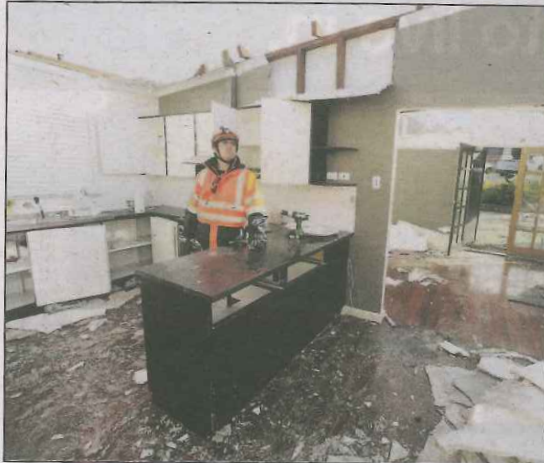
SES worker Ben Gardiner surveys the destruction in the Sutton's home after the tornado.
