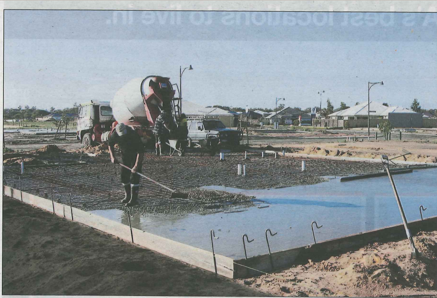
A concrete slab is poured for a new charity home which will benefit the Cancer Council WA.
